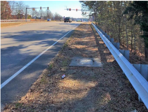
Worn path headed southbound on South Laburnum Avenue approaching the Eastbound I-64 Ramps
