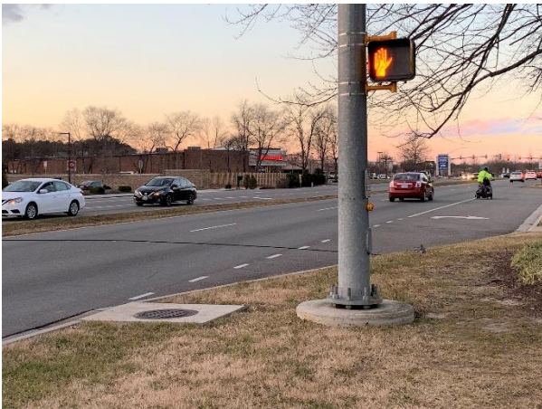
Pedestrian push button not accessible via sidewalk at Finlay Street
