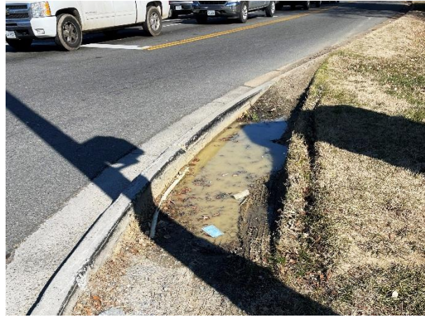
Curb damage at Audubon Drive
