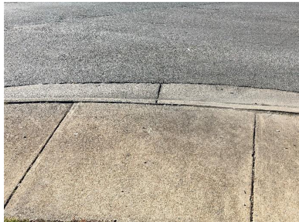
Lack of detectable warning surface on curb ramp at US 60 (Williamsburg Road)
