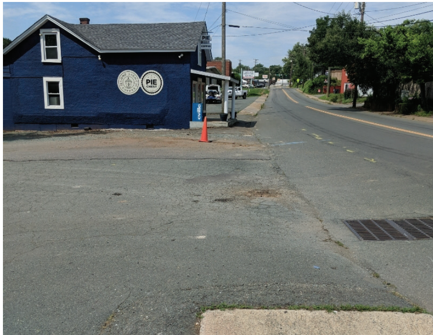
Figure 11. Disconnected sidewalk on the southeast side of East High St
