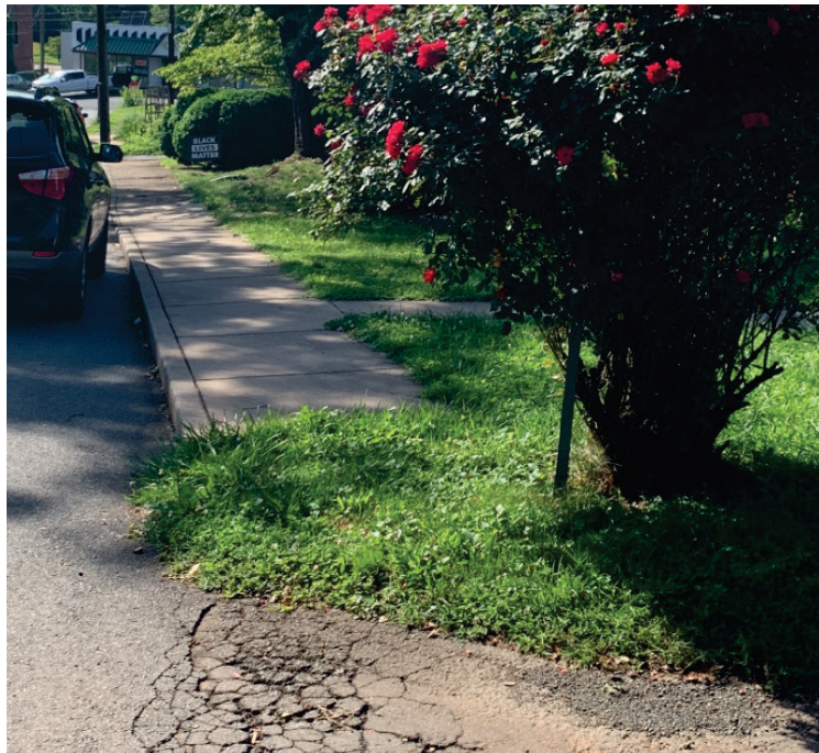
Figure 21. Disconnected sidewalk on Hazel St
