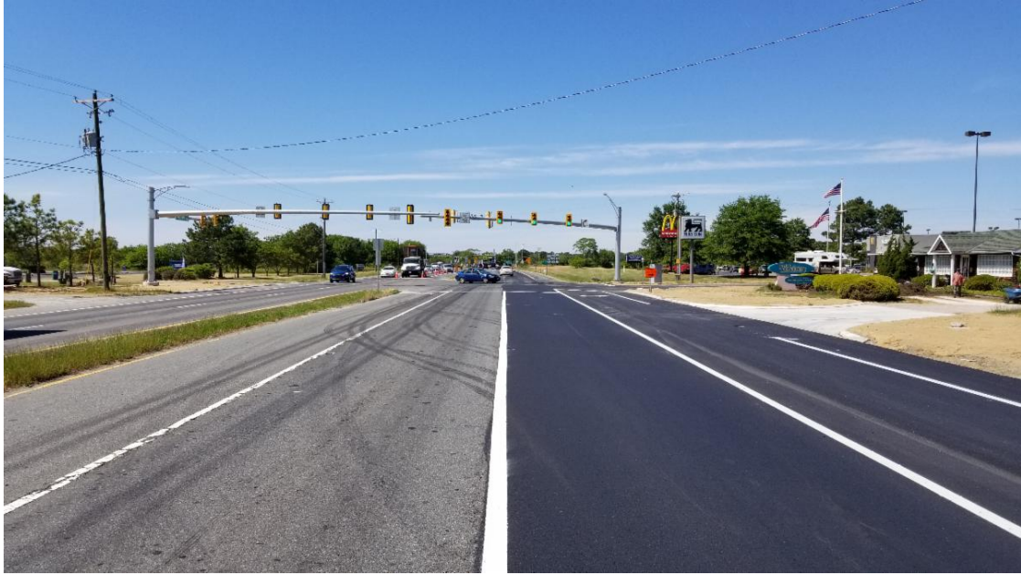
Image: View northbound on Route 13 (Lankford Highway) at the entrance to the Food Lion shopping center, with a new traffic signal placed as part of the Route 13 Improvements at Stone Road project.
